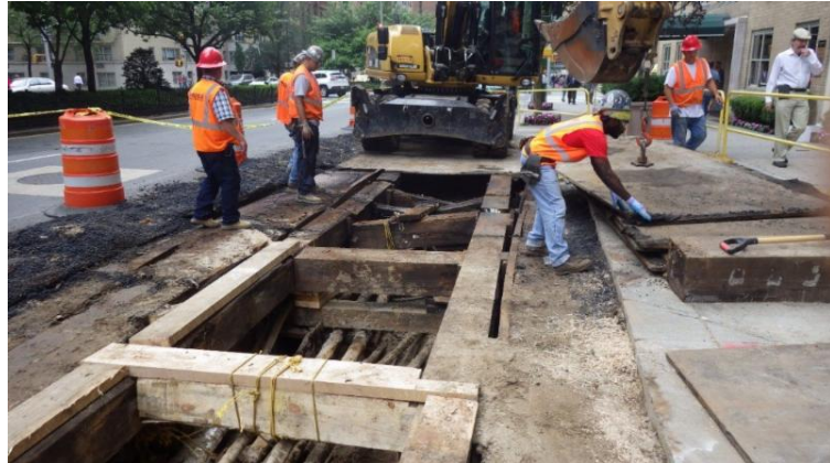
Reinforcement of the support of excavation at 37th Street and Park Avenue
