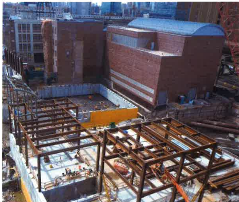
B10 Power Substation (background, right), Yard Services Building, lower foundation walls (background left), steel for future the Plaza Interlocking ventilation tower (foreground).
