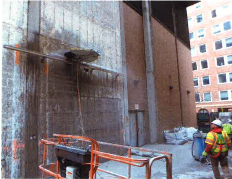
Sawcutting new equipment and material access doors at the 63rd Street & 2nd Avenue Ventilation Facility.
