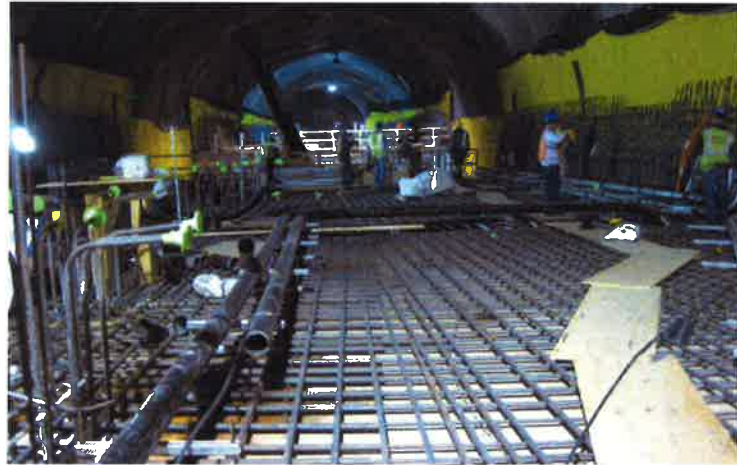
Conduit, rebar and waterproofing installation in the tunnels south of Grand Central Terminal
