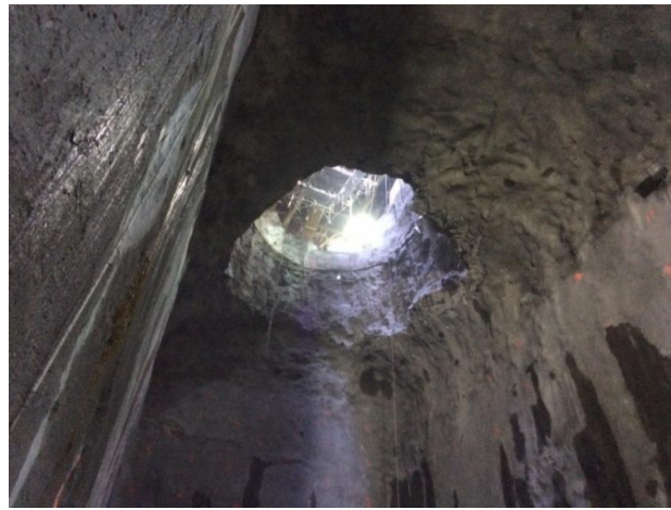
Looking up through the fully excavated air shaft from the cavern below 55th Street
