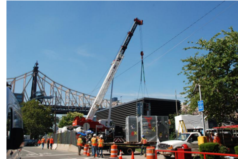
Equipment delivery at Roosevelt Island (Click the photo to view a larger version)
