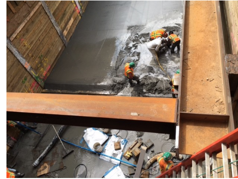
Concrete pour for West Approach (Click the photo to view a larger version)
