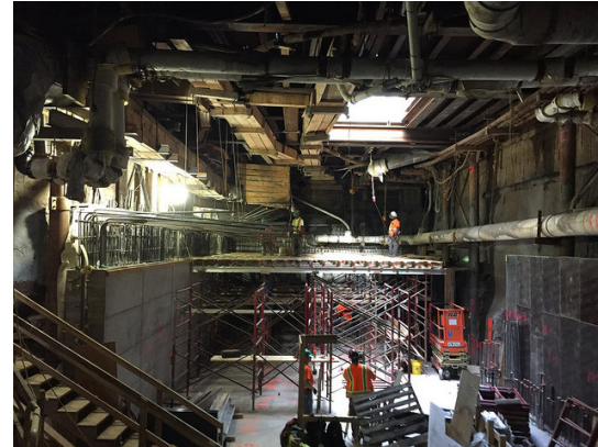
Installation of roof support below 48th Street (Click photo to view larger version)
