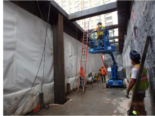
Excavation for the equipment room at 63rd Street (Click the photo to view larger version)
