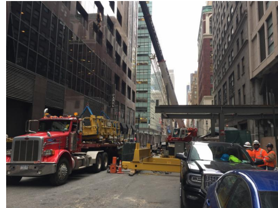
Gantry crane removal from the 44th Street vent facility (Click the photo to view larger version)
