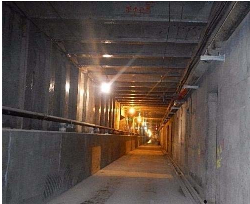
Completed concrete lining and bench installation within the eastbound 63rd Street Tunnel
