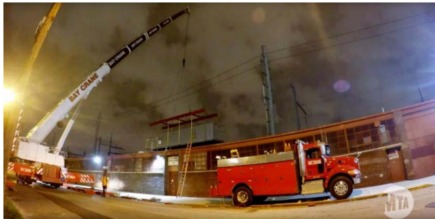
A new Central Instrumentation Location hut was installed in August along the right-of-way between 43rd and 48th Streets
