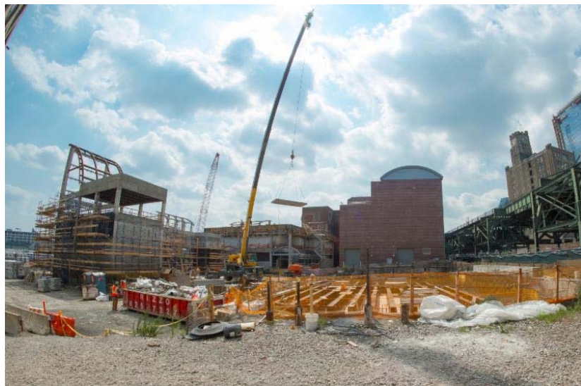
B10 Power Substation (background, right), decking over of Early Access Chamber (foreground), Ventilation Facility (background, left) and the Yard Services Building (background, center)
