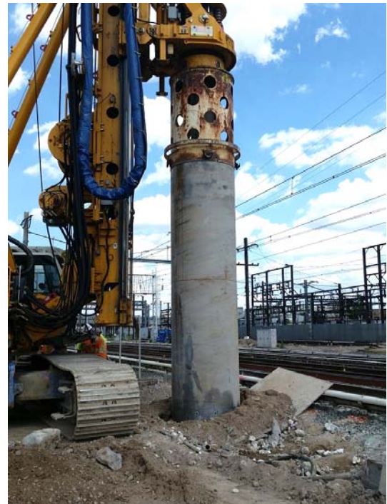
Installing a secant pile as part of the support of excavation for upcoming tunneling work
