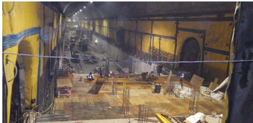
Concrete and rebar installation on the mezzanine level of the westbound cavern
