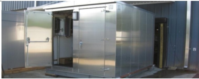
POINT Battery Hut Exterior.
