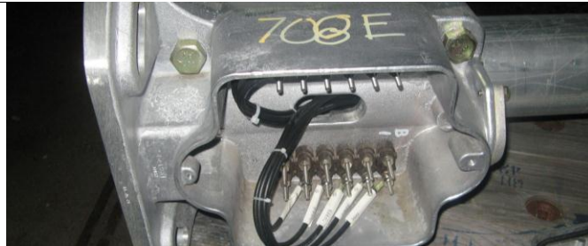
Install 708E Color Light Signal at West of F1A Signal Hut Location.
