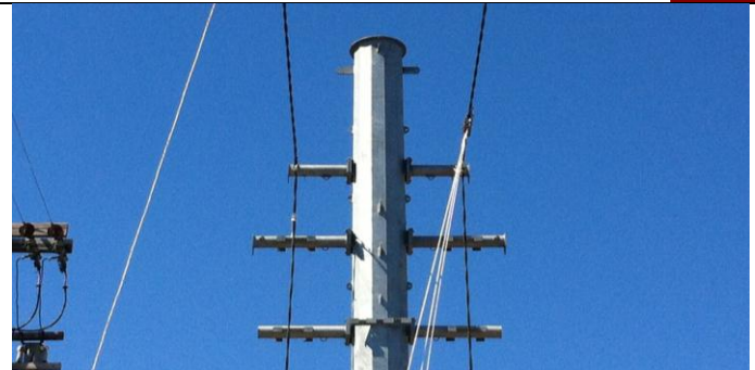
Unlashed Signal Wires at Tower 36.
