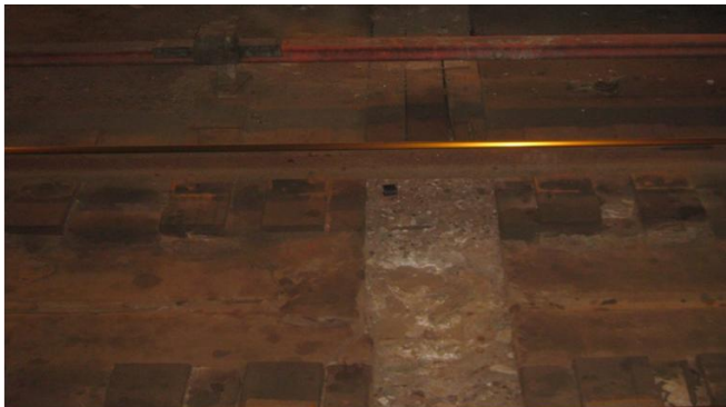
Upcoming Expansion Joint Replacement at Concrete Track Bed.
