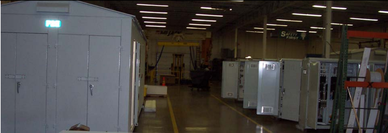
Signal Cases and F2 CIH in Amtrak Signal Facility in Lancaster, PA.
