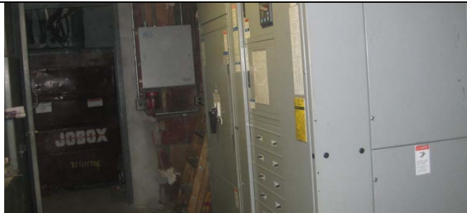
New Switchboard SB-72 in Switchboard Room D.
