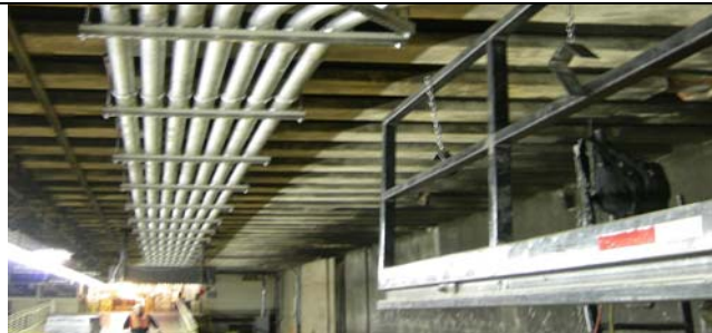
Conduits for Negative Feeders at Track 37.
