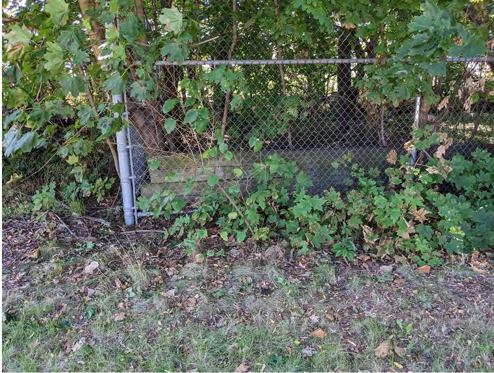
Photograph 11. Detail of the wooden retaining wall at the northeast corner of the First Methodist Church of Jamaica historic cemetery. View looking southeast.
