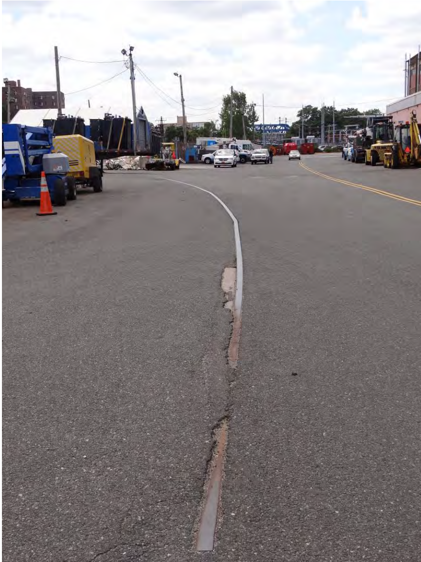
Photo 6. Former NYNH&H Railroad Van Nest Electric Locomotive Repair Shops Railroad Track, Facing West, 2013
