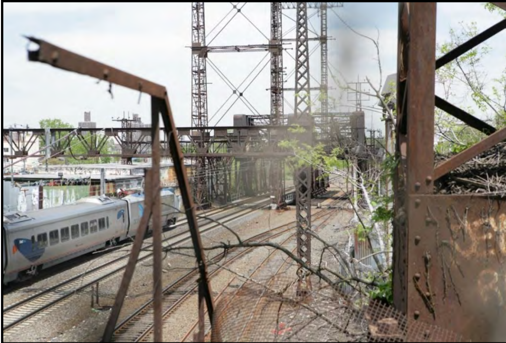
Photo 28. Amtrak Hell Gate (Northeast Corridor) Line Bascule Bridge over the Bronx River, View North. May 2013
