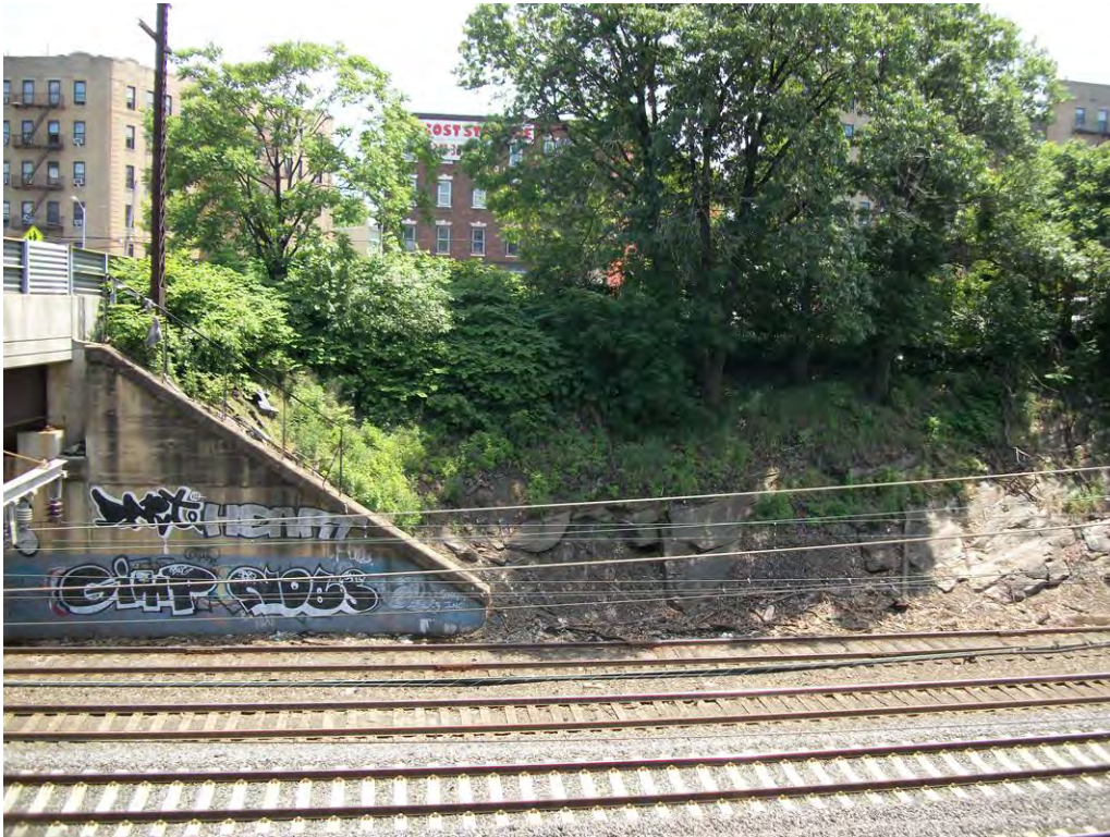
Photograph 1. Railroad cut through bedrock at proposed Hunts Point Avenue Station Site. Facing east.
