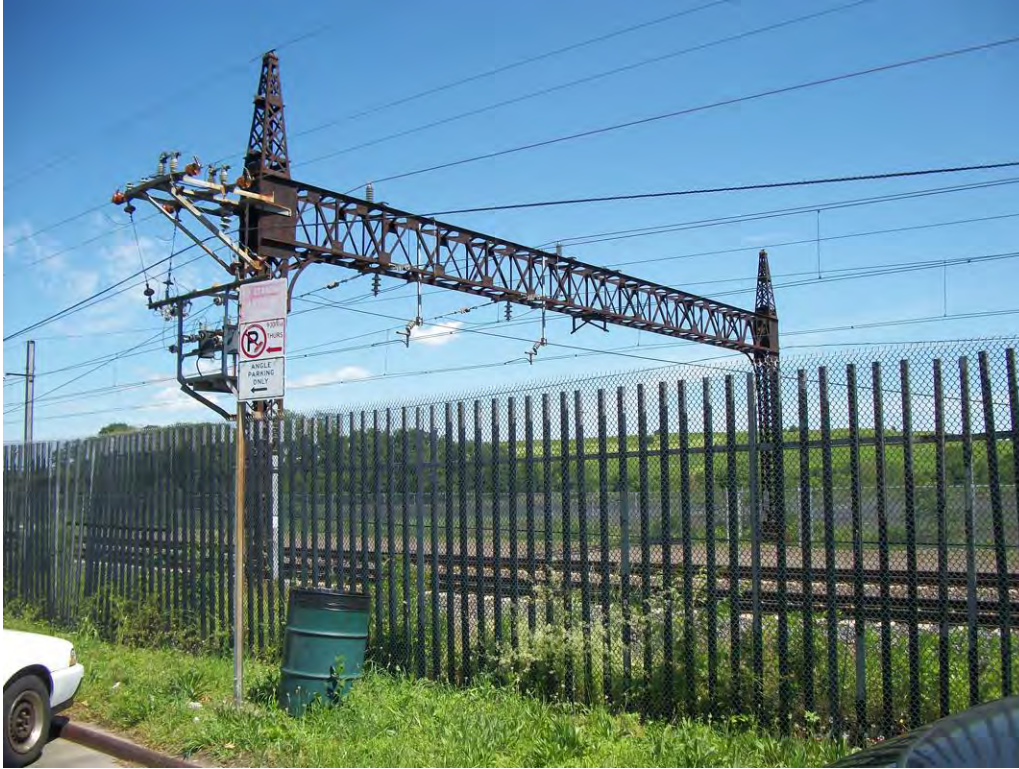
Photograph 3. Proposed Co-Op City Station location behind existing fence. Facing east from Erskine Place.
