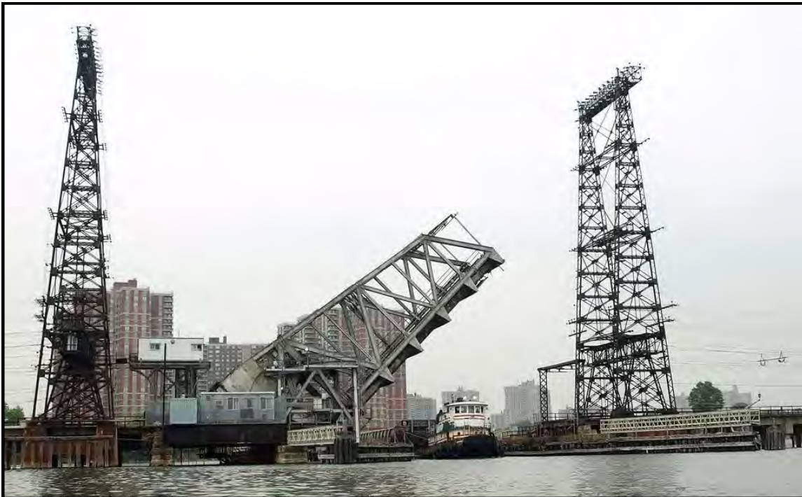
Photo 20. Amtrak Hell Gate Line (HGL) Bascule Bridge over Pelham Bay and Hutchinson River, View Northwest. May 2013
