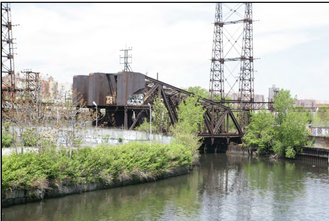
Photo 27. Amtrak Hell Gate (Northeast Corridor) Line Bascule Bridge over the Bronx River, View North. May 2013
