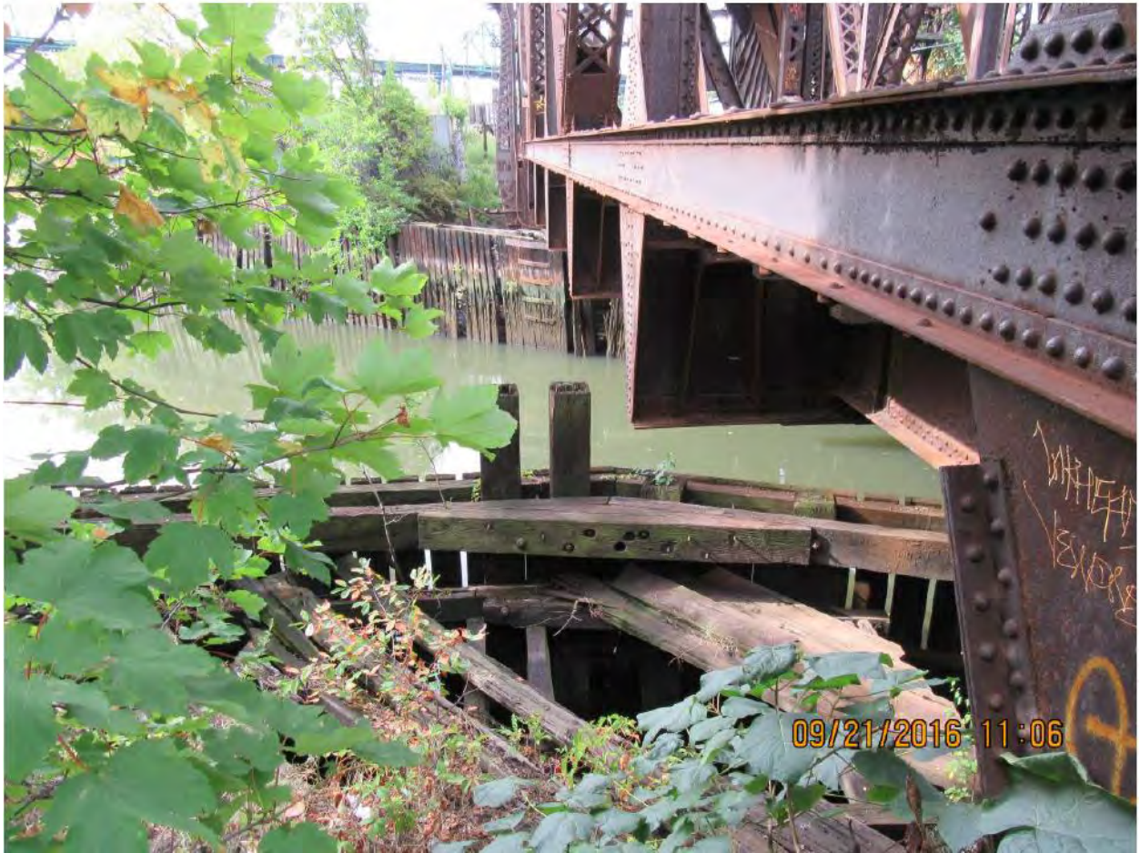
Photograph 4: Abutment beneath southwest end of bridge, facing northeast September 21, 2016 (Penn Station Access, Bridge Assessment, Bridge # 11.40 Bronx River). Note timber fender system at edge of abutment.
