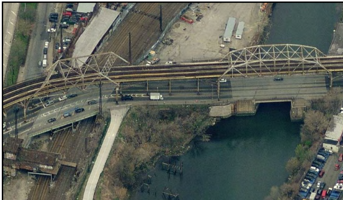
Photo 31. IRT No. 6 Subway Truss Bridge over Westchester Avenue, Amtrak Hell Gate Line (HGL) and the Bronx River, Aerial View North. May 2013
