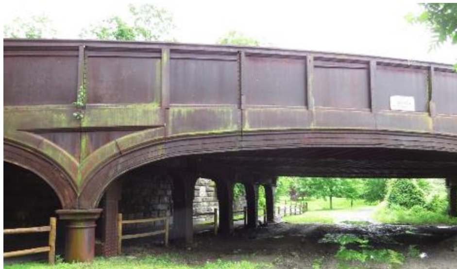
View of decorative steel piers and ornamental steel girders on north side of bridge
