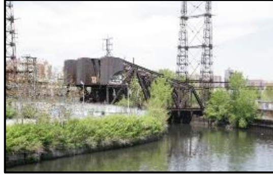
Photo 9-4. Amtrak HGL (Northeast Corridor) Bascule Bridge over the Bronx River, View North. May 2013
