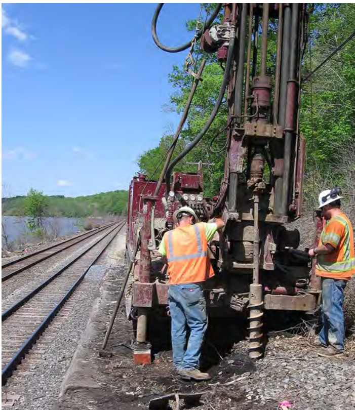
Geotechnical Exploration for rock slope stability and field support along an Amtrak line.
