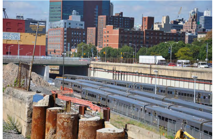
Atlantic Yards Development site is located between two of Brooklyn's busiest roadways and over nine subway lines, all of which had to remain operational due in part to experienced railroad operations specialists.
