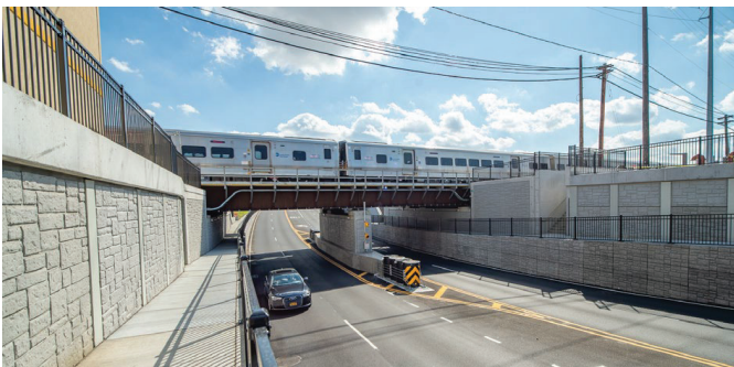
The New Hyde Park Road crossing closed on Feb 3, 2020 and reopened on Aug 24, 2020.
