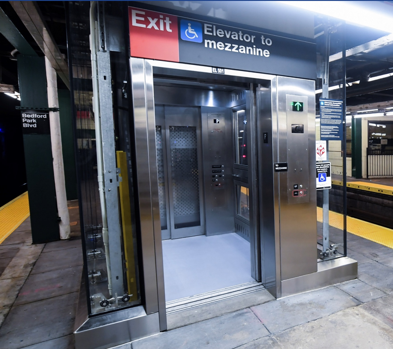
Photo: ADA Elevator at Bedford Park Blvd. - Bronx
