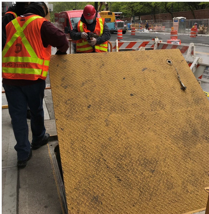
System Safety Specialist Jason Ortiz and member of the Infrastructure team conduct an inspection of an Emergency Exit.
