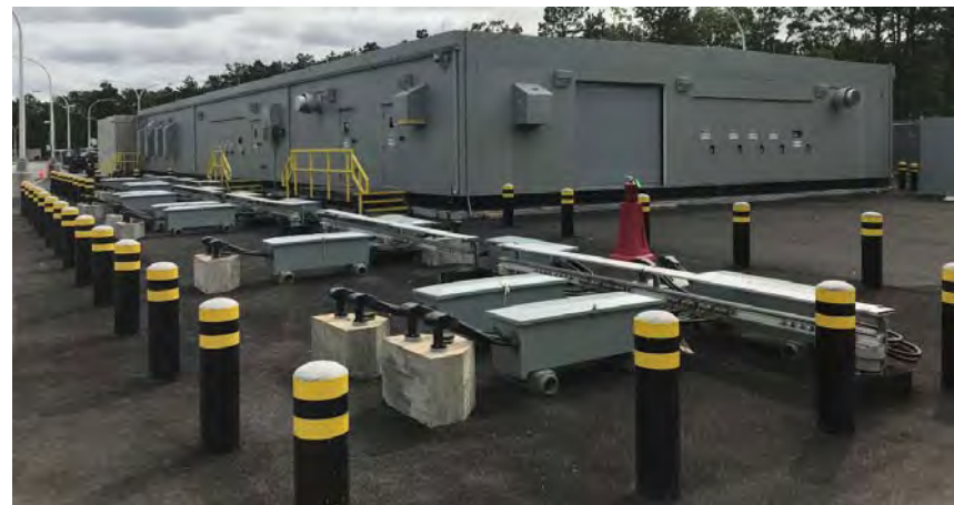
New DC Substation
