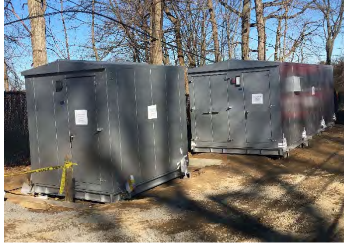
New Installed Neck 3A Signal Hut & Battery Case
