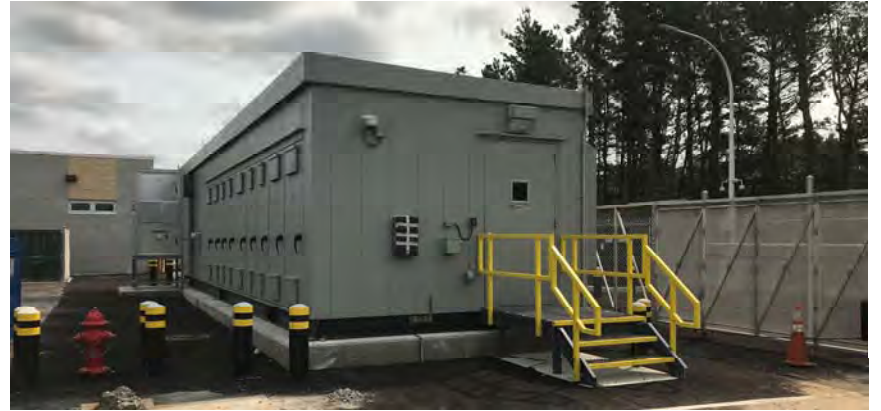
NEW AC SUBSTATION
