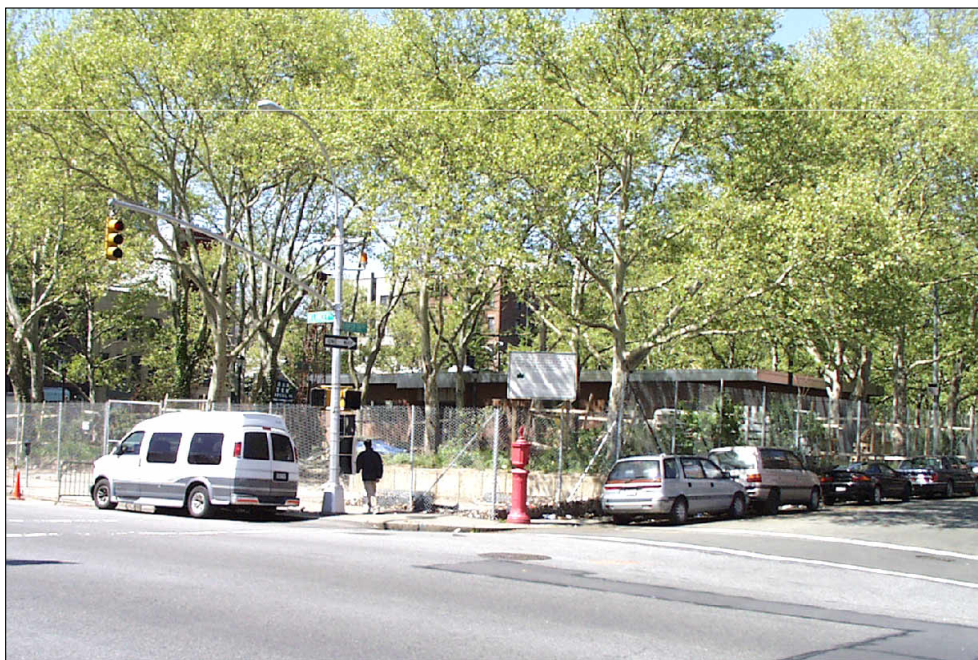
Looking northwest at soil stabilization area near senior center from Delancey Street 4
