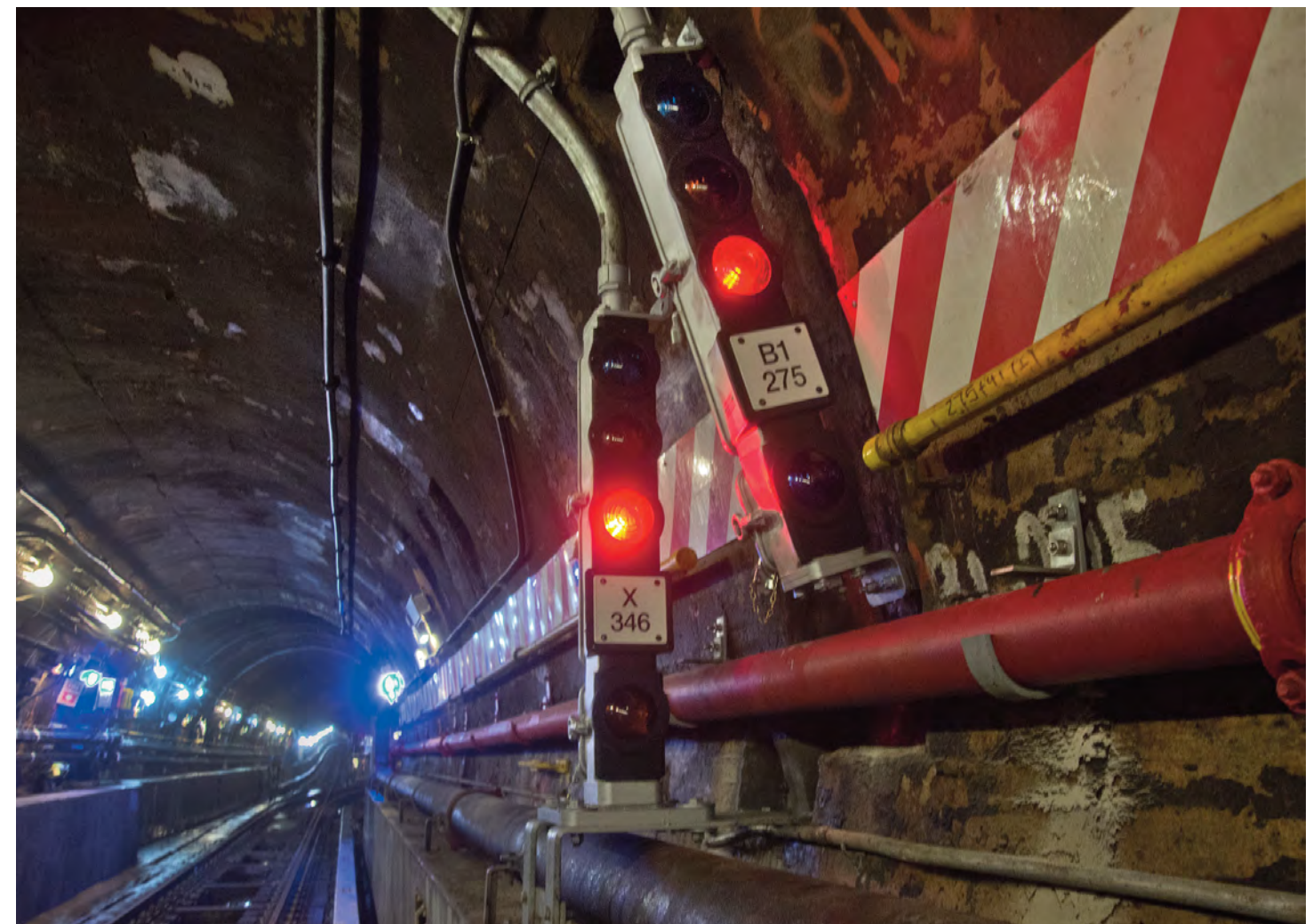
Top, L to R: Post Sandy damage, Damaged circuit board, Repair of damaged infrastructure Center, L to R: New cables running through duct banks, New pump room, Repair of damaged tube Bottom: Tube, post repair
