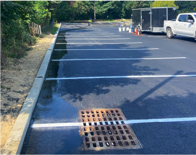
Drainage at the Speonk Station parking lot regularly back-up into the lot and onto existing property.
