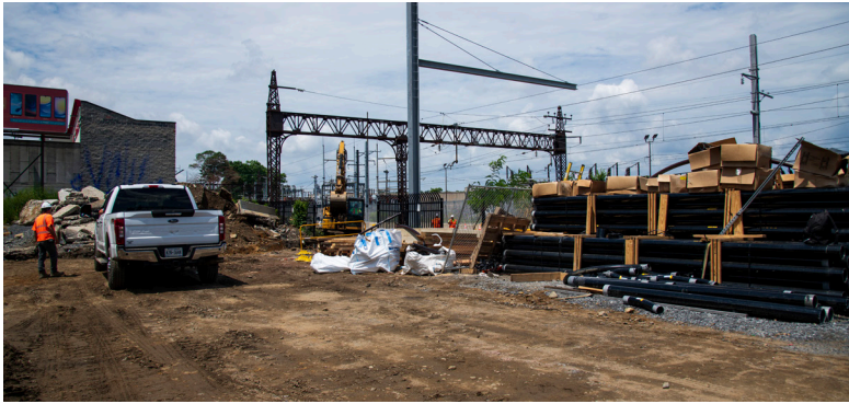
Above: New and preexisting OCS portals at site of future Parkchester/Van Nest Station, July 2024
