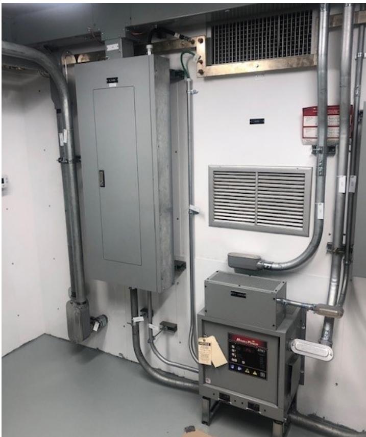
Inside look at the Mobile Substation, which provides consistent signal power while replacement work is underway.
