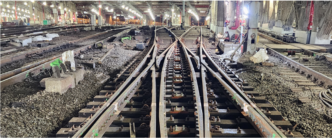
Repairs to West Side Storage Yard started this month, which was damaged during Superstorm Sandy
