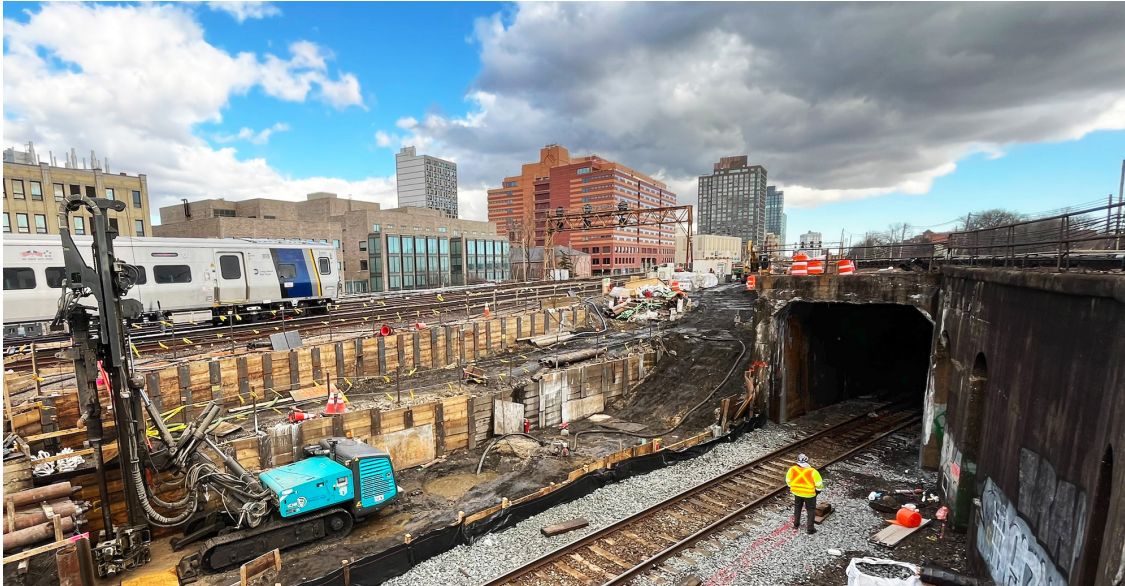
Crews prepare the area around Jamaica Station to make way for capacity improvements.
