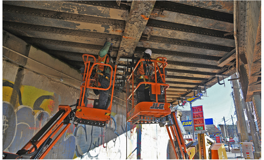
PSA construction workers preparing for superstructure demolition work at Bronxdale Avenue Bridge, December 2023
