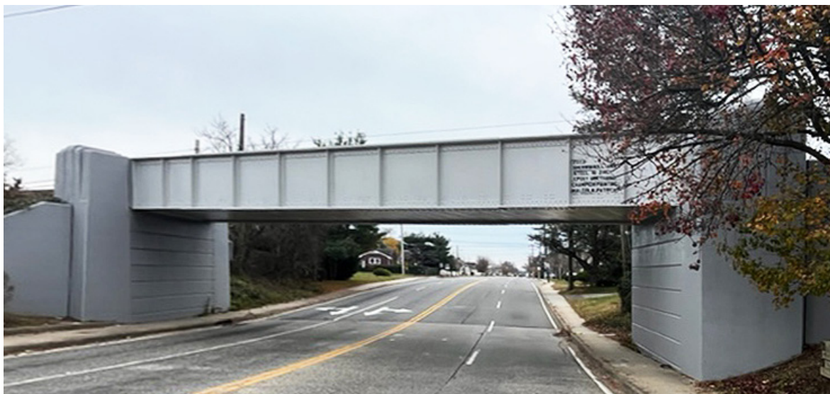
Merritts Avenue Bridge is one of eight LIRR bridges that has been repainted as part of state-of-good-repair efforts.
