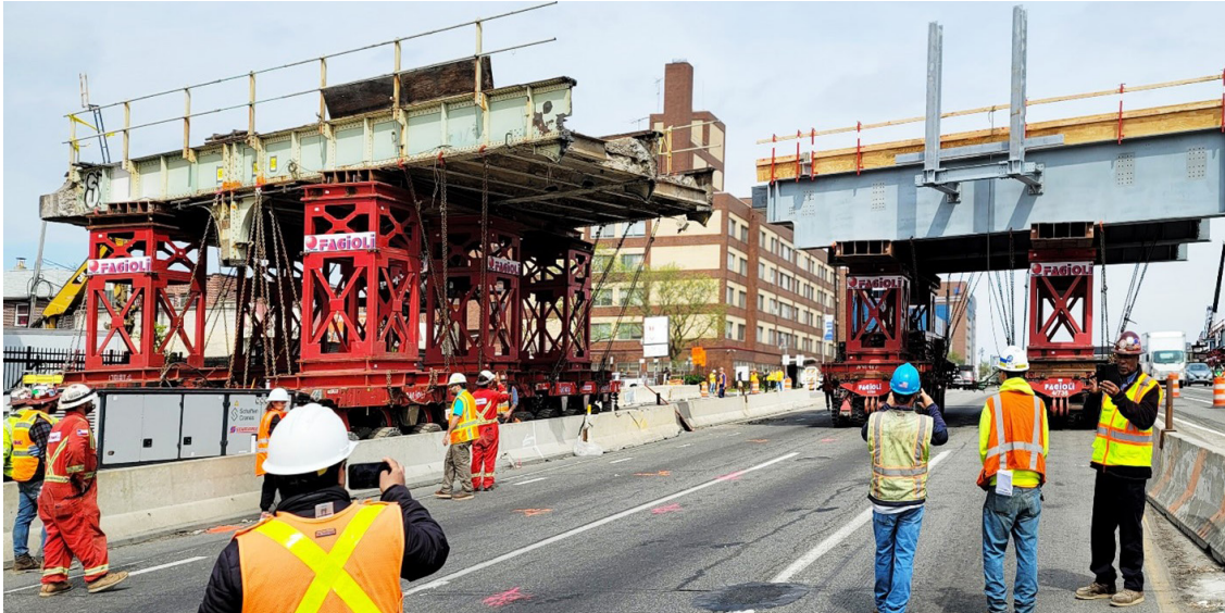
Crews look on as a new bridge over the Van Wyck Expressway is rolled into place.
