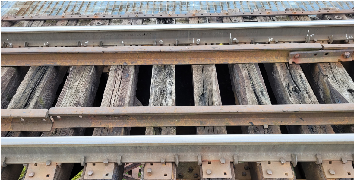
Up close of the timber ties on the Moodna Viaduct in Orange County, which are being replaced.
