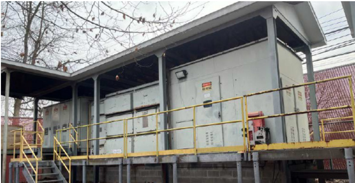
The decades-old Pelham Substation will be replaced with a new, more resilient facility.
