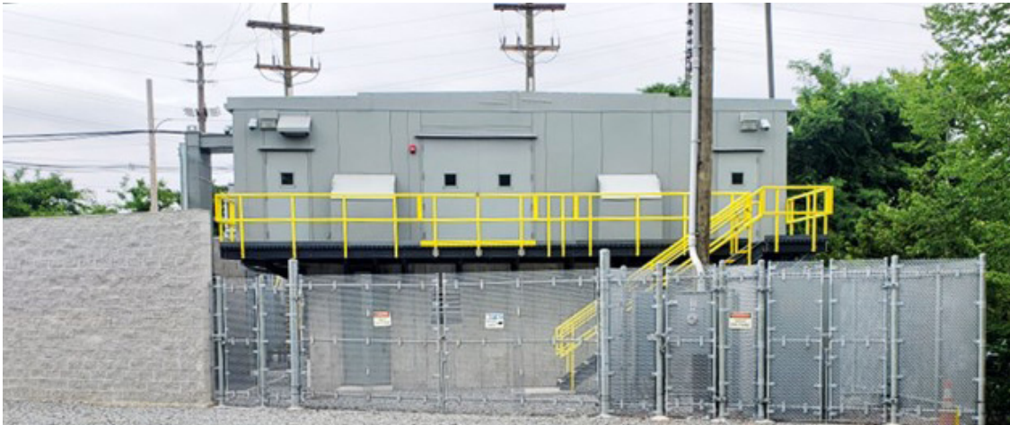
The new Ocean Avenue substation improves the reliability of LIRR power infrastructure.
