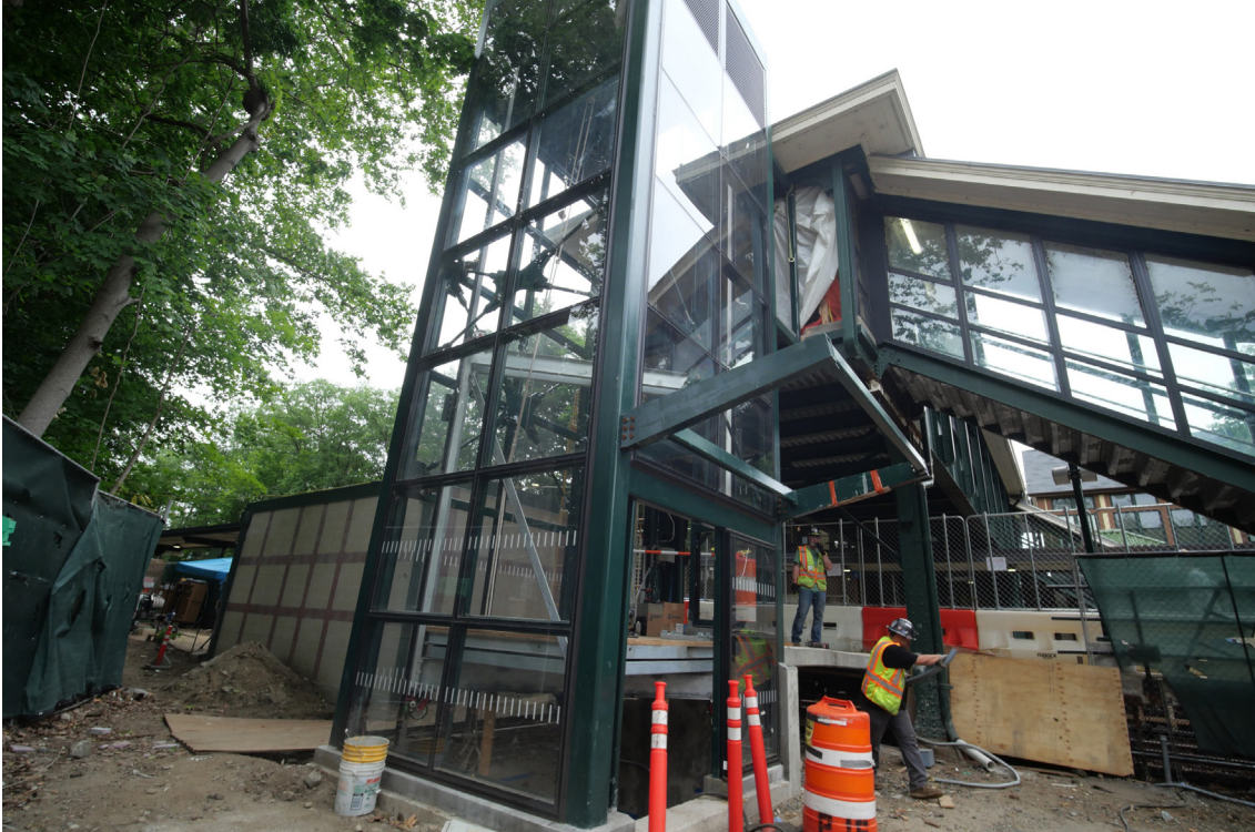
A new elevator is being constructed at Scarsdale Station on the Harlem Line.
