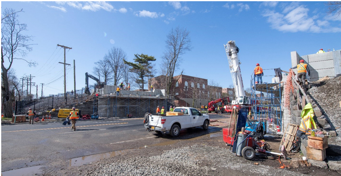
LIRR worked closely with the Village of Garden City and Nassau County to ensure replacement of the Cherry Valley Avenue Bridge replacement proceeded smoothly
