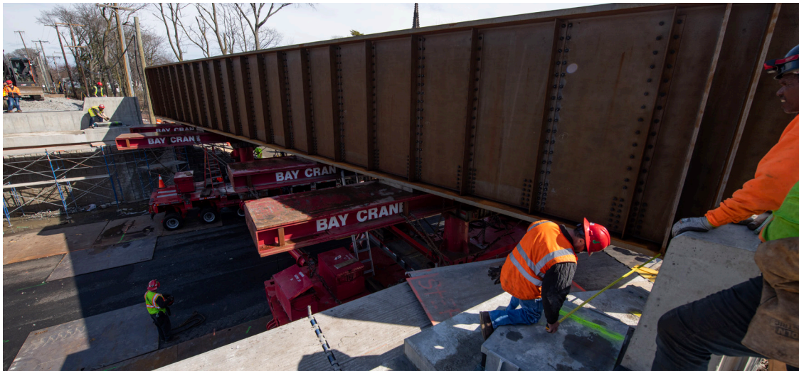
Crews prepare to install the new Cherry Valley Avenue Bridge in Garden City
