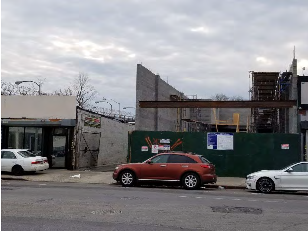
Photograph 17: Lot 76 showing new building under construction. View looking southwest from Merrick Boulevard.
